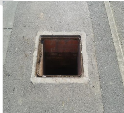
Missing Chamber Cover
